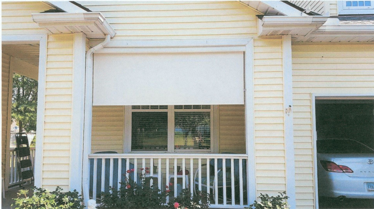
Solar shade in open position
